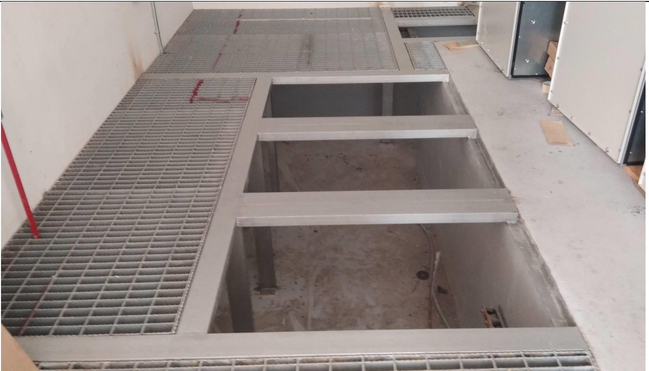
Project: Pearl Bay Mix Development Project-City of Lights, Al-Reem Island, Abu Dhabi Consultant: ACG- Architectural Consulting Group Main Contractor: Malaih Investment & Projects Development LLC Description: Hoist Access Door & Gi Grating at Sub-Station
